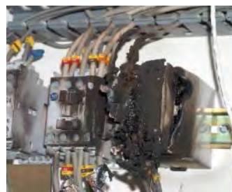
Fig. 16. Failure in switch box caused by current harmonics
